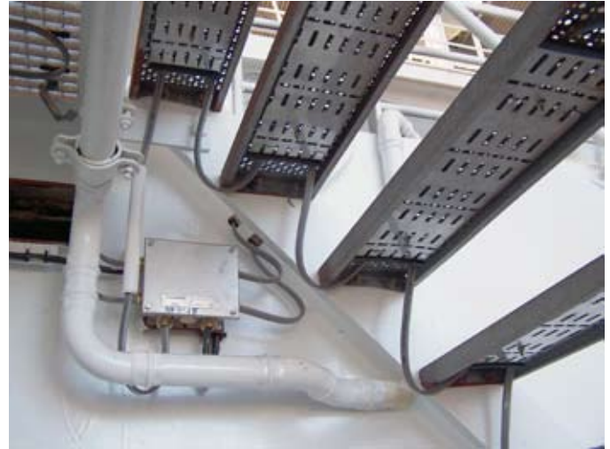
Photo 5: Heating Cable installed below stair grating, with junction box shown..
