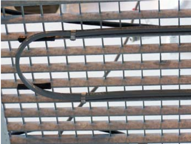
Photo 4: Heating Cable installed below open deck grating.
