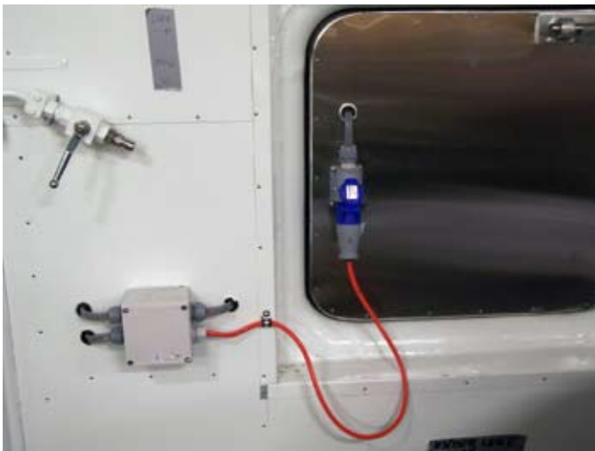
Photo 6: Door with Heating Cable installed, junction box shown.
