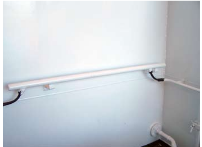
Photo 3: Heating Cable installed inside a handrail.
