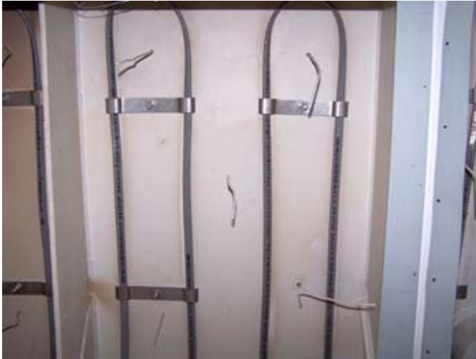
Photo 1a: Heating Cable installation on flat surface utilizing brackets with spot-welded bolts.
