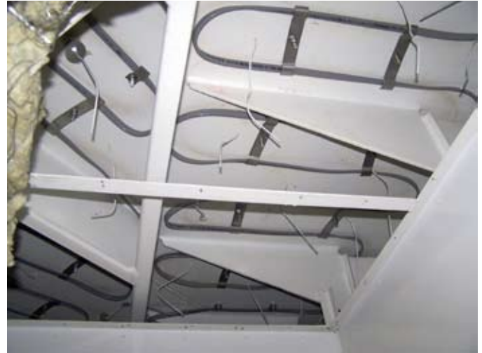
Photo 1b: Heating Cable installation on flat surface utilizing brackets with spot-welded bolts.
