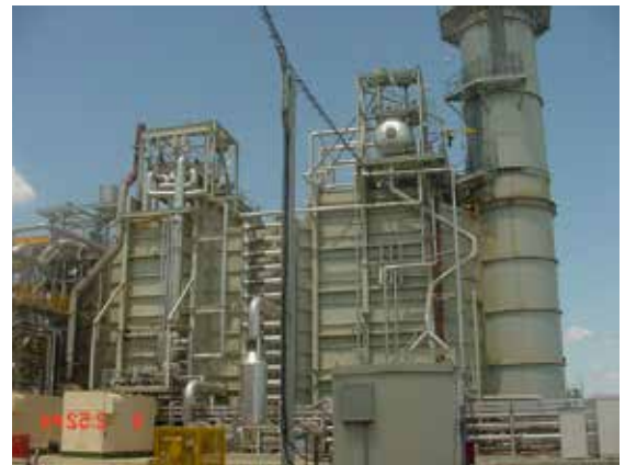
Typical HRSG units capture Combustion Turbine exhaust to generate steam. This is most often used for additional power generation.
